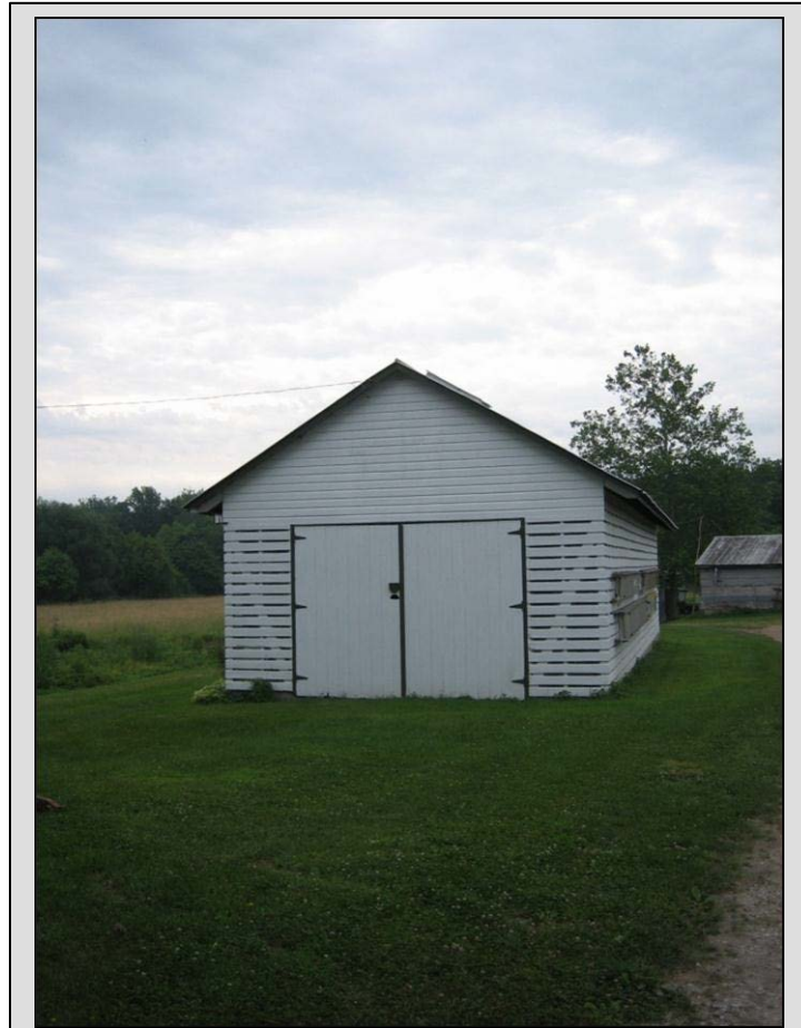
Drive-through machinery shed and corn cribs, Butler Township, Adams County. Site 001-BU-006.
