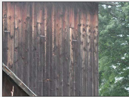
Close-up of hinges on a tobacco barn, Cowanesque River Valley, Deerfield Township, Tioga County, c. 1900. Site 117-DE-001.
