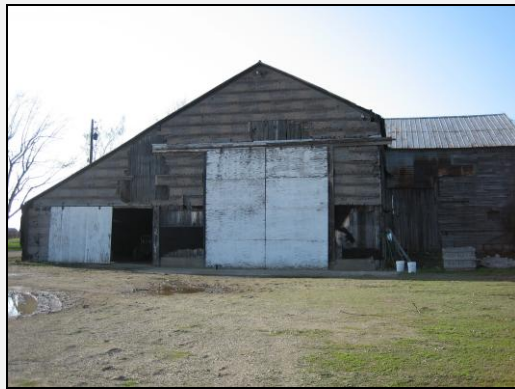
Grape packing barn extension, North East Township, Erie County, c. 1950-60. Site 049-NE-005.
