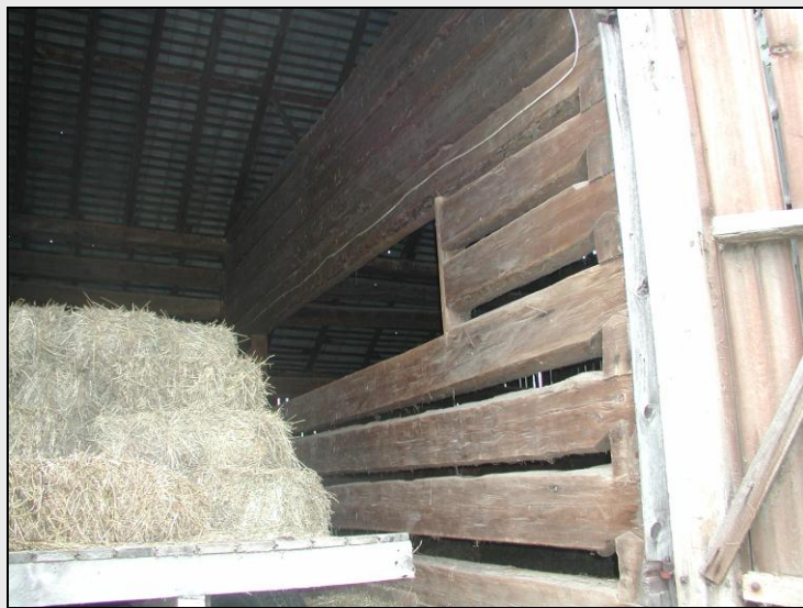
Interior log crib, Dunlop barn, Potter Township, Centre County, early 19th century. Photo only site, no site number.
