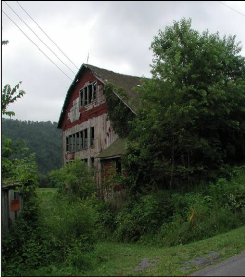
Pennsylvania Forebay barn converted for poultry, Lower Mahanoy Township, Northumberland County, original barn c. 1875, alterations c. 1950. Site 097-LM-002.
