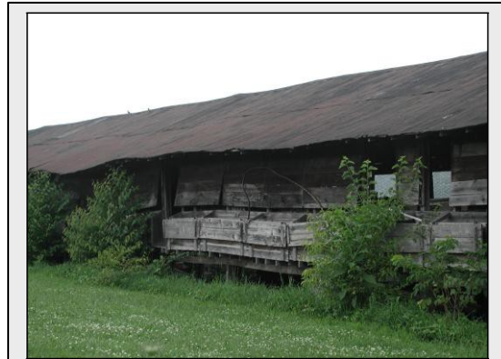
Pole barn showing nesting boxes, Lower Mahanoy Township, Northumberland County, c. 1950. Site 097-LM-003.
