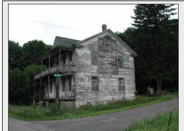
Five-bay, center passage house, Lower Mahanoy Township, Northumberland County, c. 1850. Site 097-LM-002.
