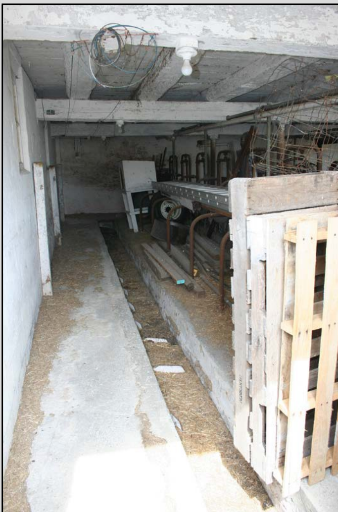
Pennsylvania Barn interior under enclosed forebay showing concrete floor, manure gutter, metal stanchions, and metal framed windows, Washington Township, Franklin County. Original construction late nineteenth century, adapted for dairy in the twentieth century. Site 055-WA-003.
