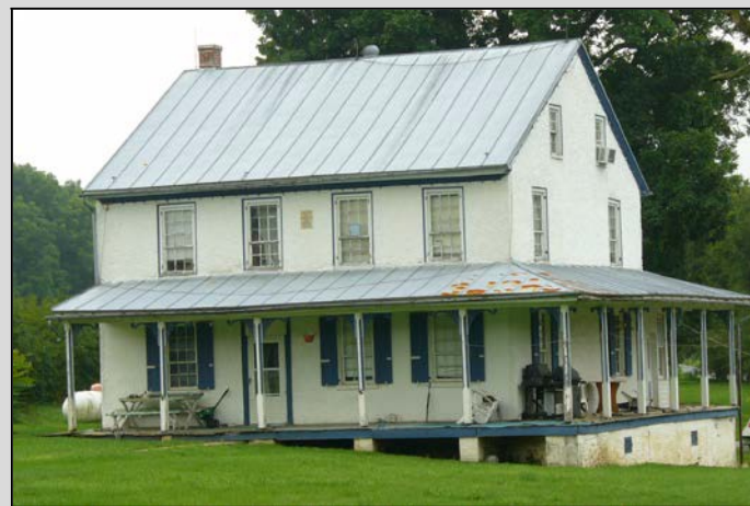
Four over four house with one door, Mill Creek Township, Lebanon County, 1843. Site 075-MC-008.
