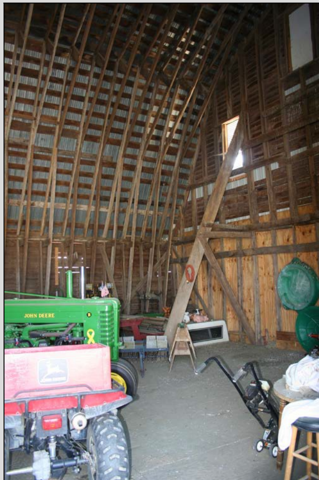
Interior framing, barn at site 055-LU-001. Note the light, short members and lack of posts.
