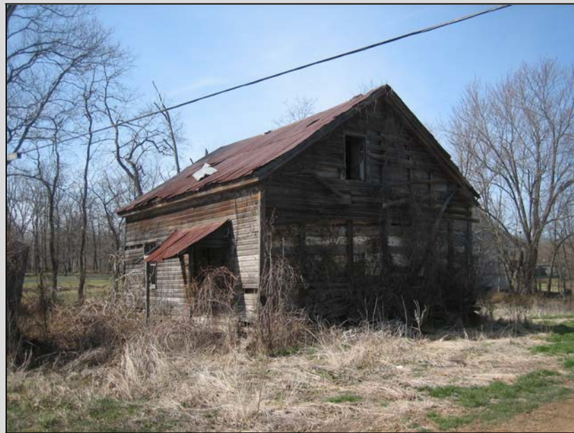
Log tenant house, Antrim Township, Franklin County, early to mid-nineteenth century. The house has a three-room floor plan. Site 055-AN-009.
