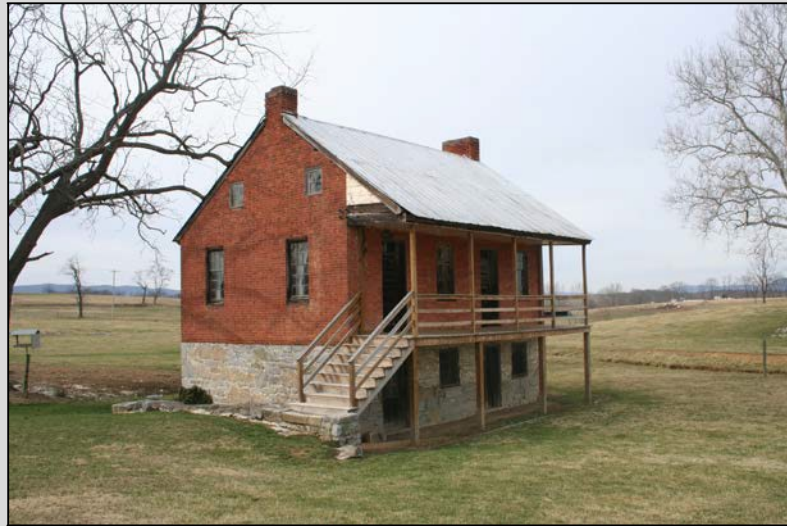
Ancillary house, possibly a tenant house, Montgomery Township, Franklin County, early to mid-nineteenth century. Site 055-MO-004.
