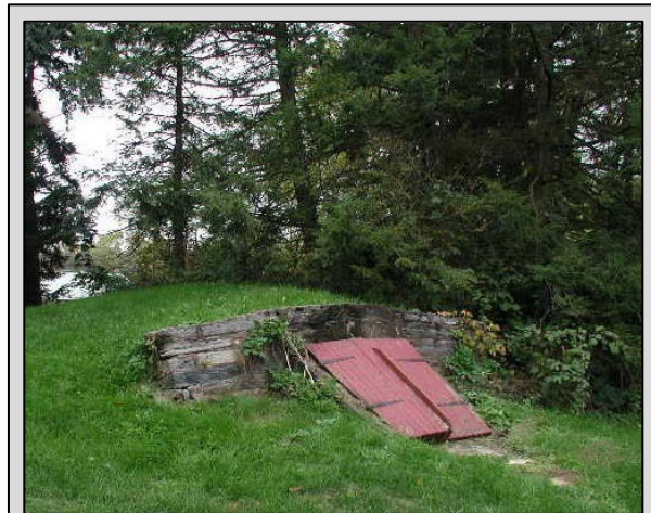
Root cellar, Schaefferstown, Lebanon County, date unknown. This cellar has a vaulted ceiling.
