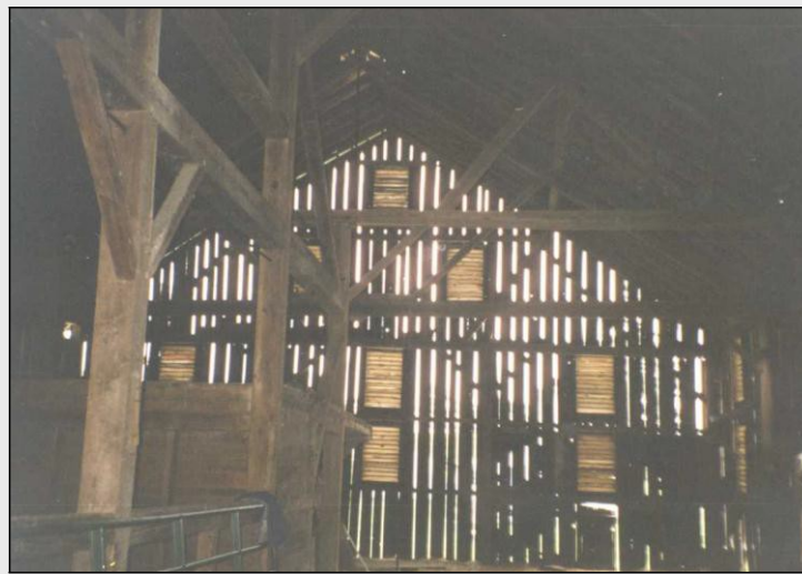
Three-gable barn interior, Potter Township, Centre County, c. 1880-1900. Photo-only site, no site number.
